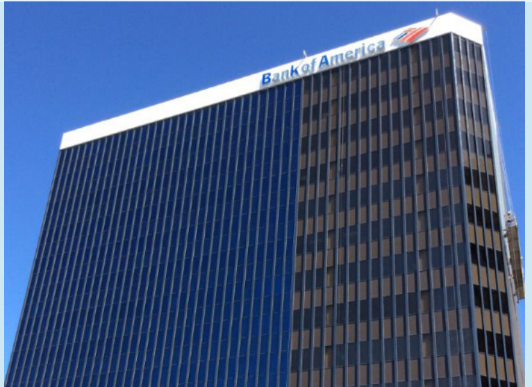
Project during installation – the original reflective bronze glazing can be seen on the right, and the subtle, sophisticated shade of AzuLite 35 Xtra on the left.
